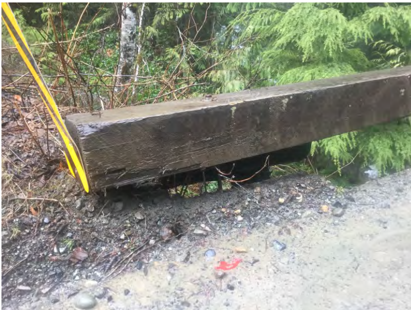
Missing riser and only 1 bolt
