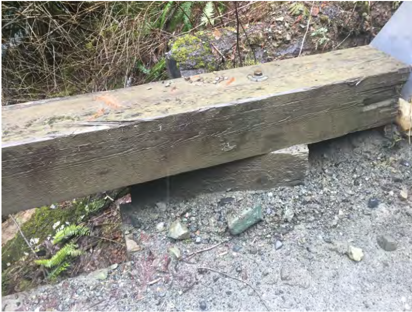
Missing bolt on guardrail
