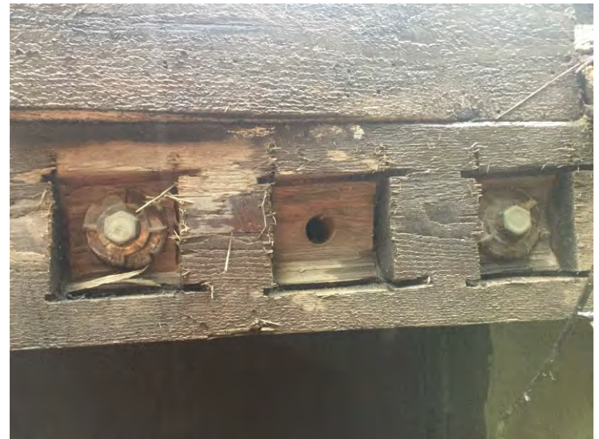
Missing block bolt and rotting
